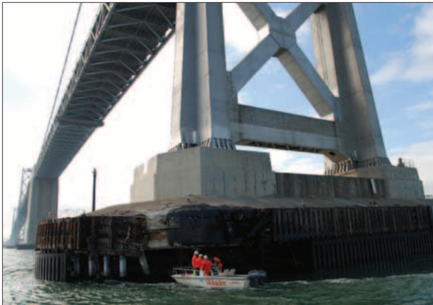
▲ From USCG 11th District Public Affairs, bridge damage survey video, Delta pylon fendering.
